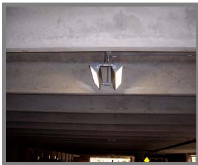
Twin Housing Unit-1 ballast
